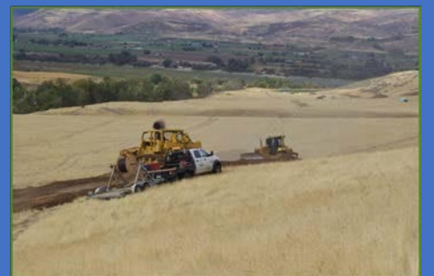
Photos courtesy of Rusti Lattin Eagle Telephone System, Inc.
